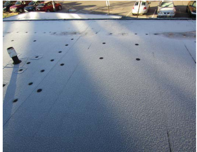
Figure 6: Membrane roof, illustrating thermal leaks at points of attachment.
