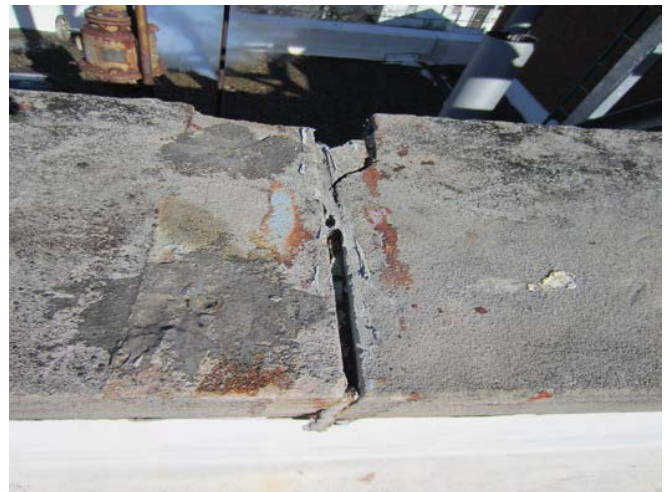
Figure 8: Cracked and broken coping, open joint resulting from mortar and sealant failure.
