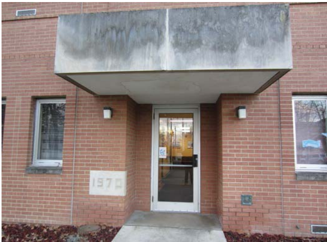
Figure 3: Masonry stains and open mortar joints at entry
