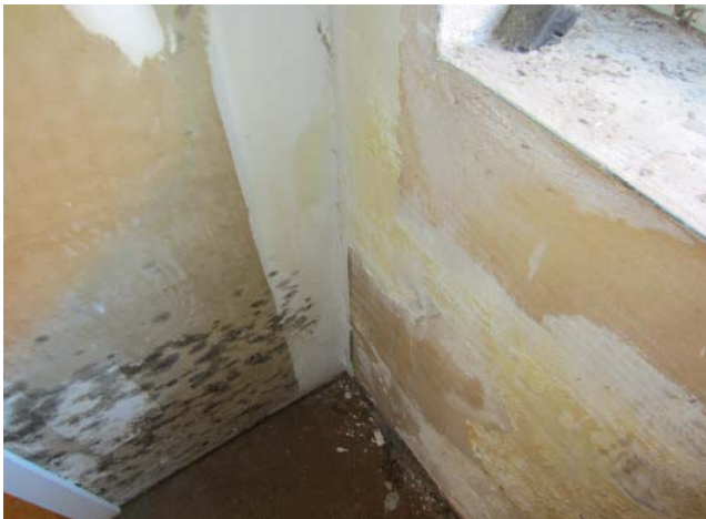
Figure 3: Possible moisture infiltration damage at basement
