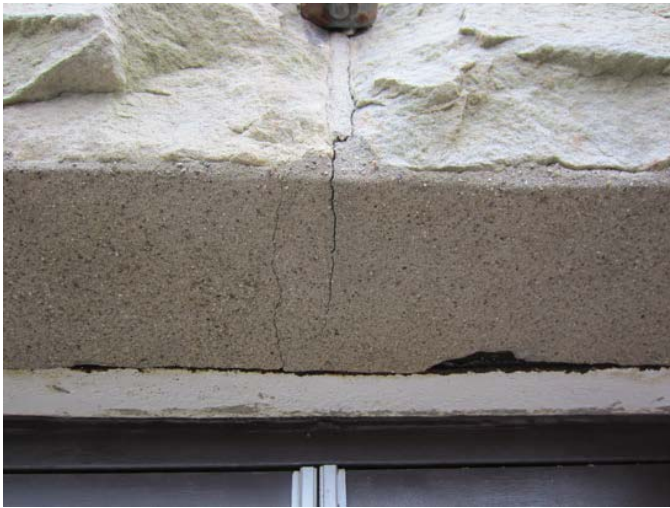
Figure 5: Crack in concrete repair to stonework, above doorway.
