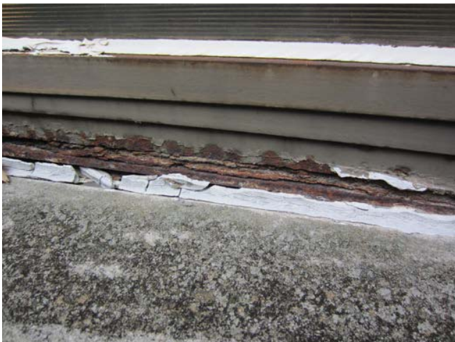
Figure 7: Window frame corrosion and sealant failure at sill
