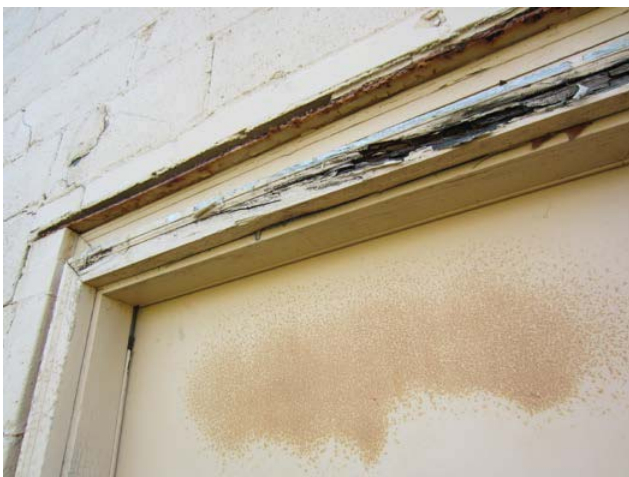
Figure 3: Exterior door corrosion and frame deterioration
