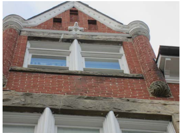
Figure 4: Cracked masonry and mortar loss on east facade
