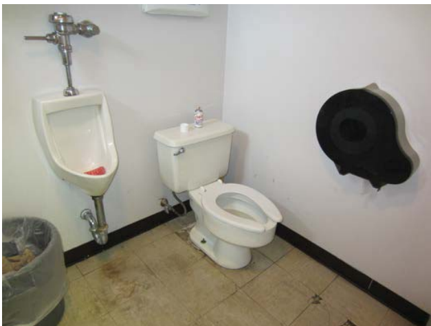
Figure 3: Damaged floor finish at toilet room
