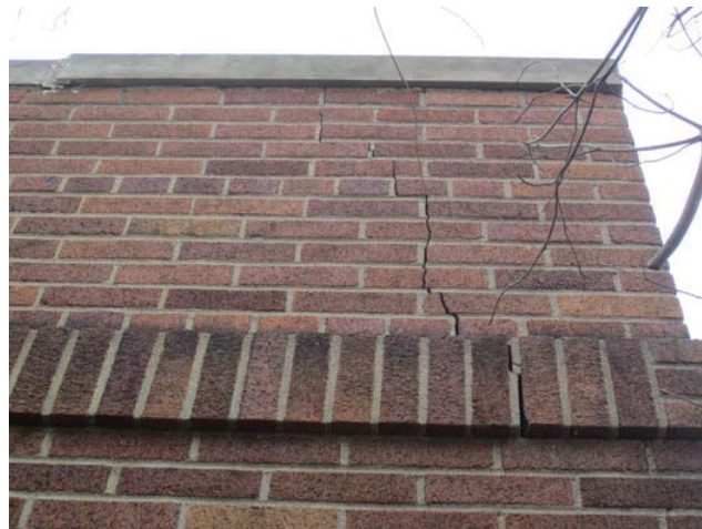
Figure 2: Cracked masonry and open mortar joints (typical)
