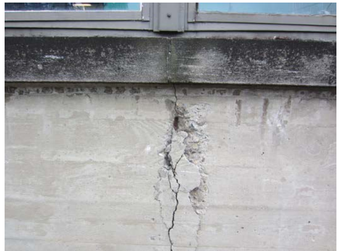
Figure 6: Cracking and spalling of concrete
