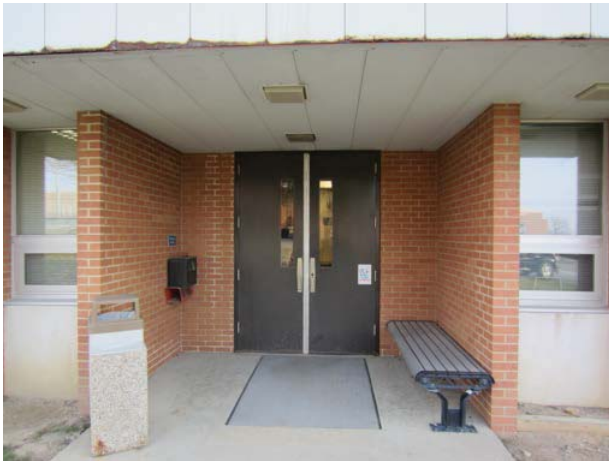
Figure 3: Canopy Corrosion at Entrance
