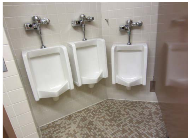
Figure 8: Non-compliant fixture clearances for accessibility. Cracked, broken wall tile.
