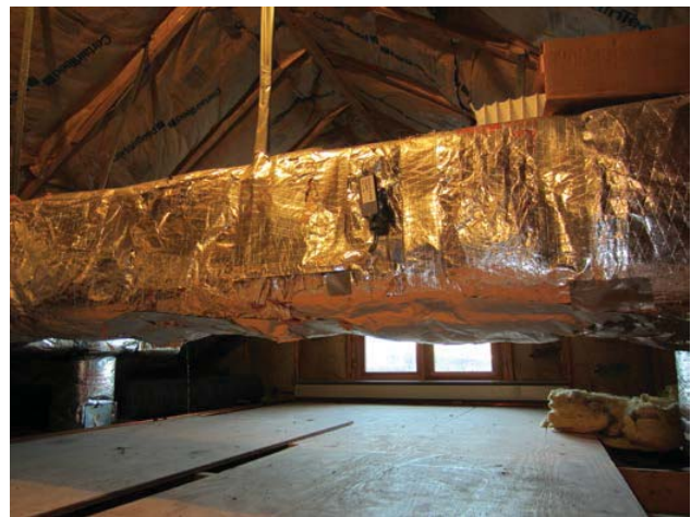
Figure 4: Attic interior with distribution ductwork
