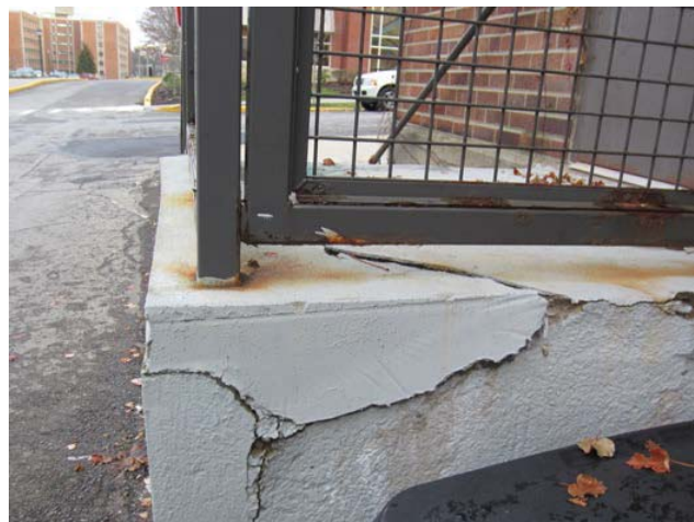
Figure 4: Concrete spalling at entrance
