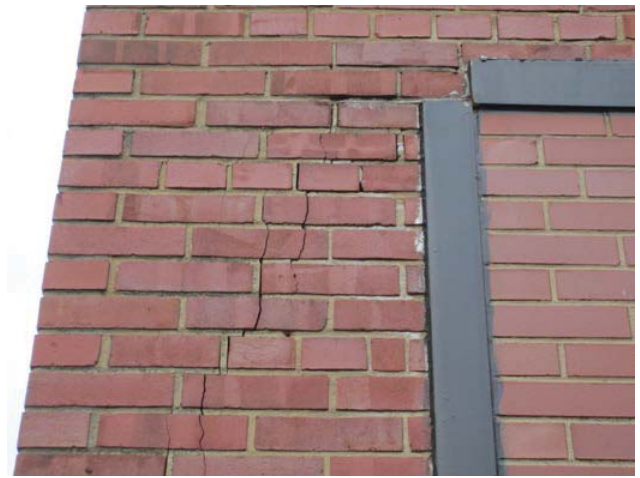
Figure 4: Cracked brick masonry and mortar
