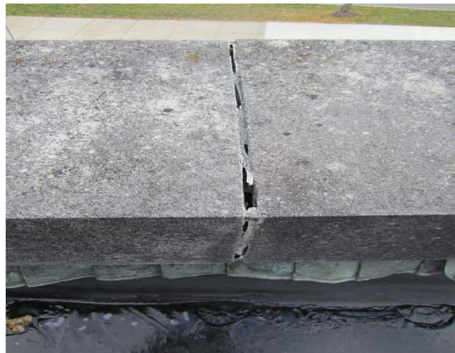
Figure 6: Sealant failure at limestone coping
