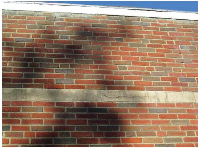
Figure 2: Cracked brick and mortar, spalling cast stone
