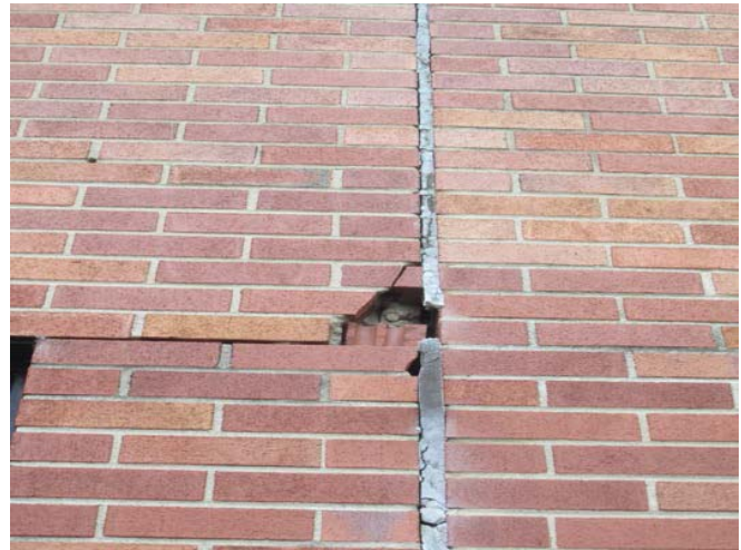
Figure 6: Sealant failure at expansion joint, with masonry spalling and cracking.
