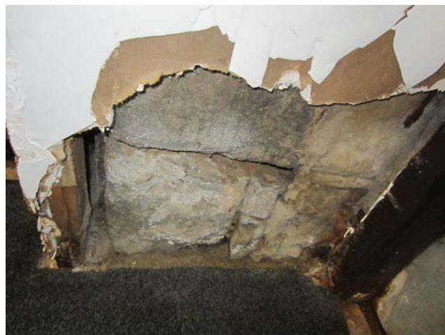
Figure 4: Moisture damage and corrosion at entry
