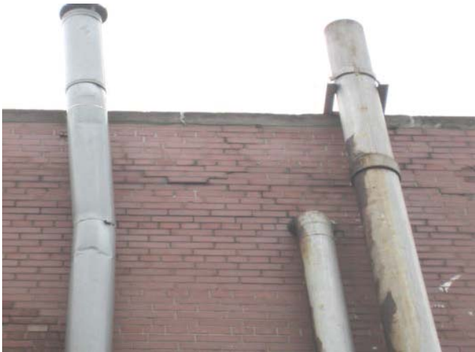
Figure 5: Masonry cracks and brick displacement
