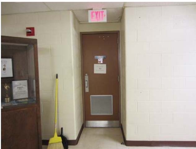
Figure 7: Non-compliant clearances at toilet room entry for accessibility
