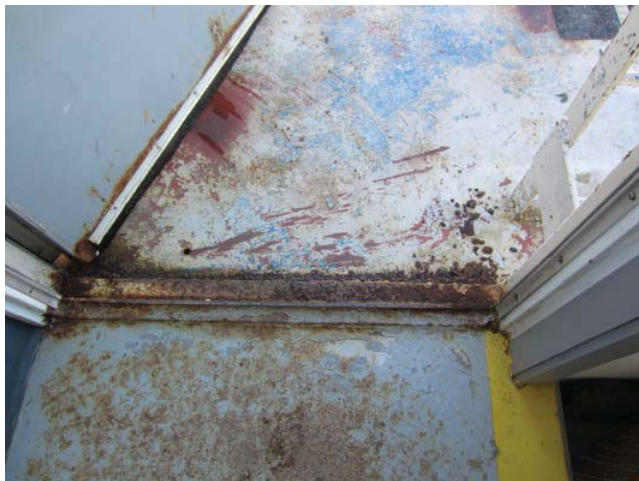
Figure 3: Corrosion at pressbox entrance
