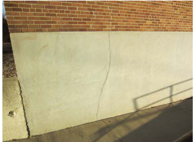
Figure 2: Cracking at foundation wall, south facade
