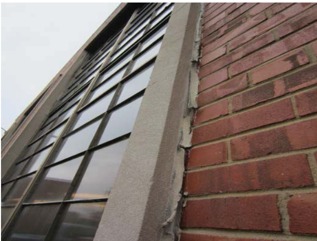
Figure 3: Sealant failure between limestone and brick masonry
