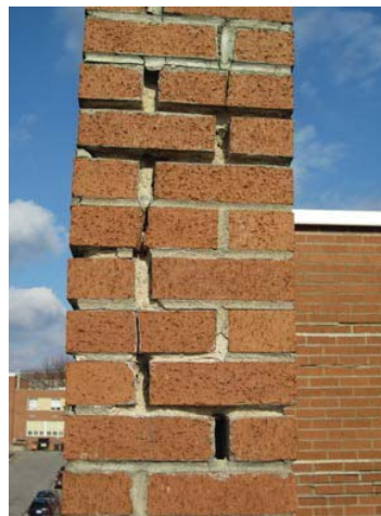
Figure 4: Masonry condition at screen wall
