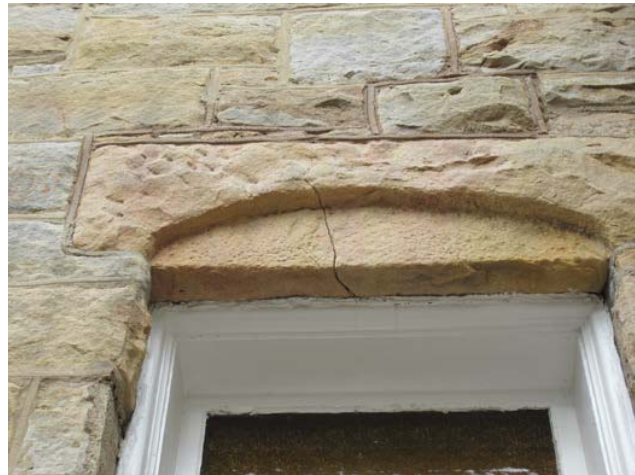
Figure 2: Cracked stone lintel
