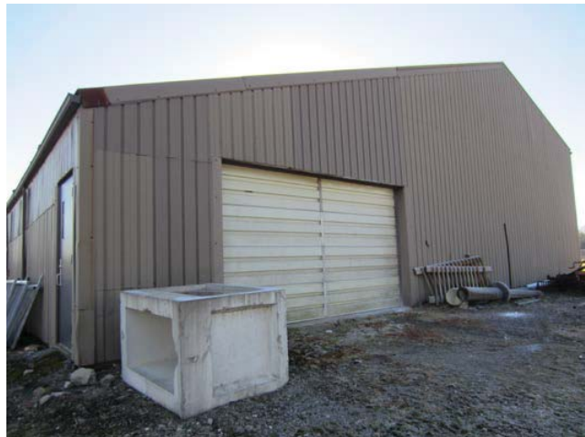
Figure 2: Exterior corrosion at roof flashing and impact damage at wall panels
