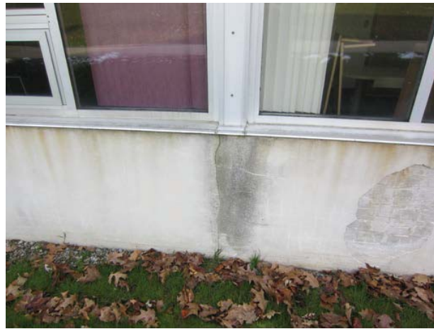
Figure 2: Cement Plaster Cracking and Spalling
