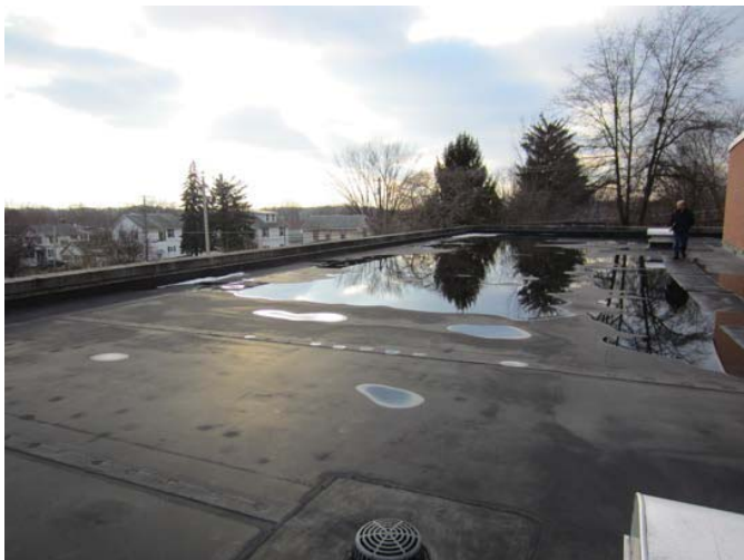
Figure 5: Roof water ponding
