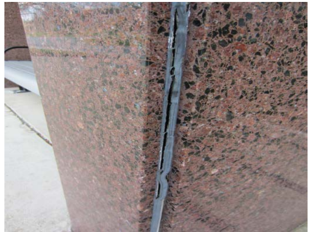
Figure 4: Sealant failure at marble panel joint
