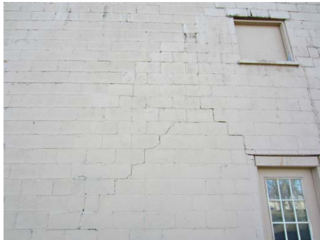
Figure 2: Cracked concrete masonry (typical)
