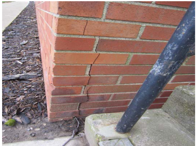
Figure 4: Cracks in brick masonry
