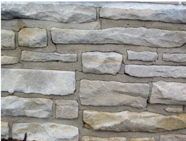
Figure 3: Cracks in stone masonry
