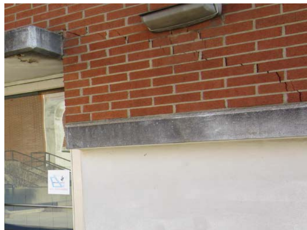
Figure 4: Cracks in brick masonry and mortar
