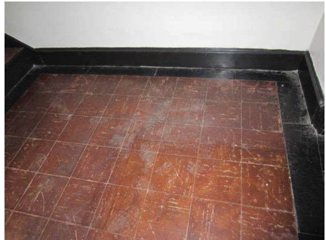
Figure 4: Possible asbestos floor tile at stair landing
