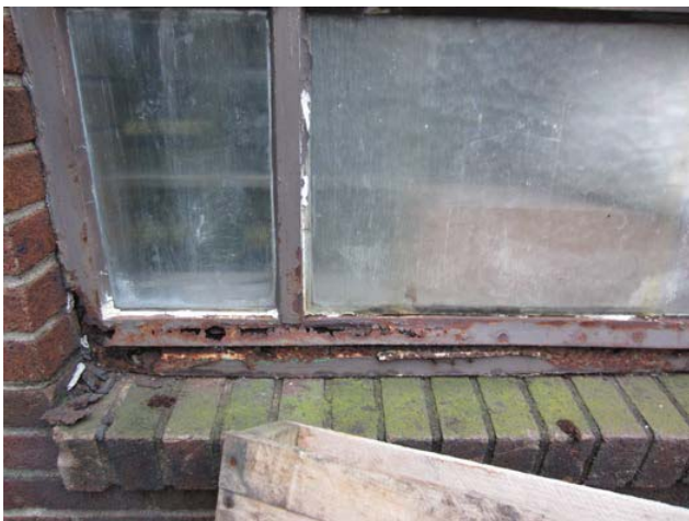
Figure 3: Window frame corrosion
