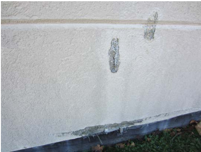
Figure 5: Stucco damage at building exterior
