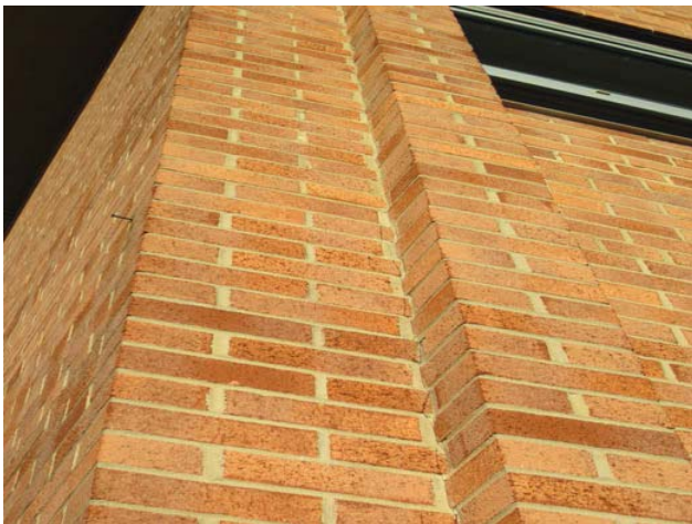
Figure 3: Vertical crack at inside corner of masonry, southeast corner of building
