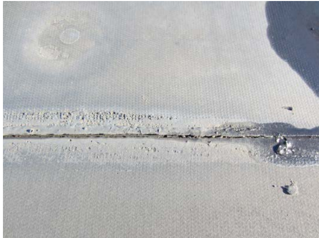
Figure 6: Deterioration at roof membrane seam
