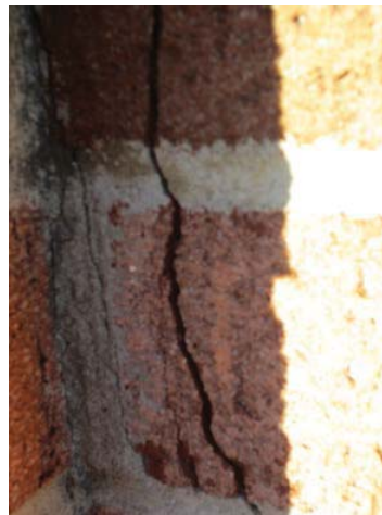
Figure 4: Cracked brick masonry on east facade
