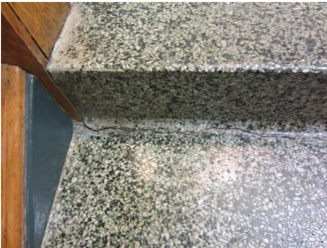
Figure 5: Cracked terrazzo stair finish in atrium
