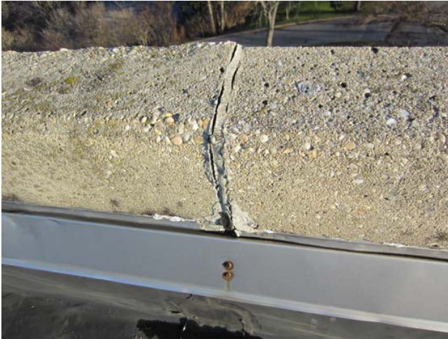
Figure 5: Spalling and sealant failure at roof coping
