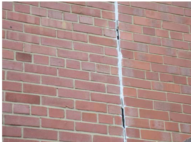
Figure 2: Sealant failure and open joint in masonry at expansion joint
