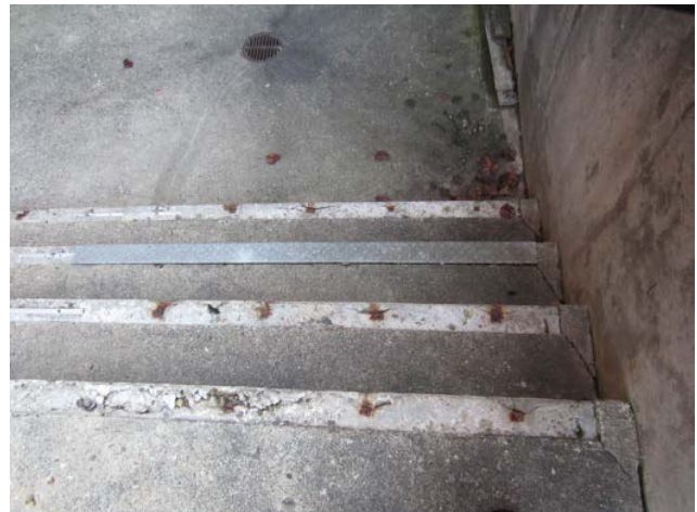
Figure 4: Cracking and spalling at concrete steps, broken and missing steel nosings.
