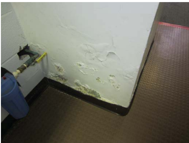
Figure 3: Moisture damage at basement level
