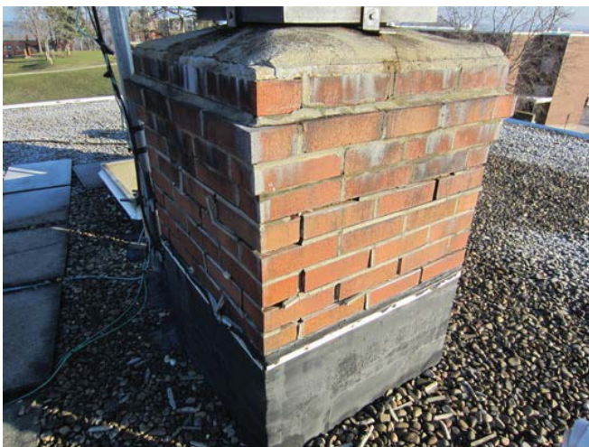
Figure 7: Open joints and cracks in chimney masonry
