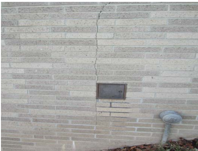
Figure 3: One of multiple vertical masonry cracks
