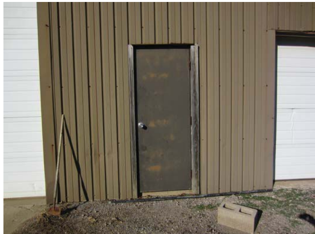
Figure 4: Door, hinge and wood jamb deterioration at hollow metal entrance.
