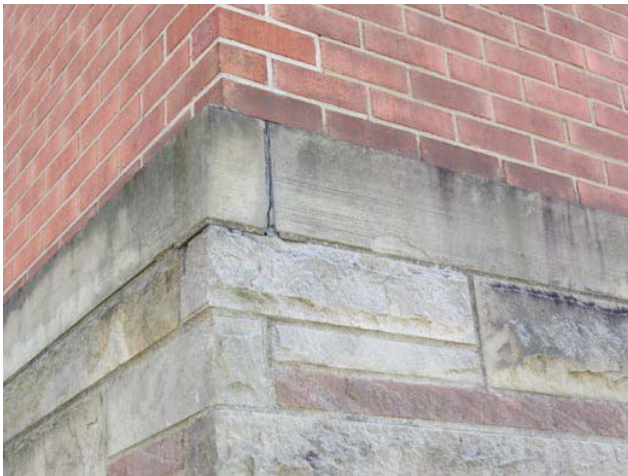
Figure 3: Mortar cracks at ashlar stonework
