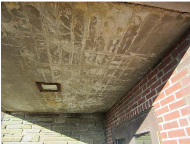
Figure 3: Concrete soffit corrosion at entrance
