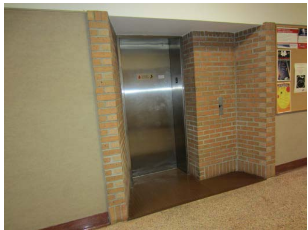
Figure 4: Elevator entrance cut into corridor construction
