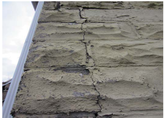
Figure 2: Cracked masonry and open mortar joints (typical)
