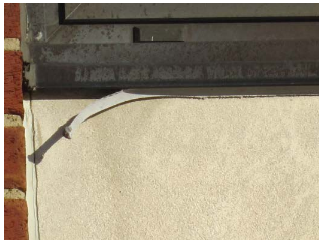
Figure 4: Sealant failure at limestone panel
