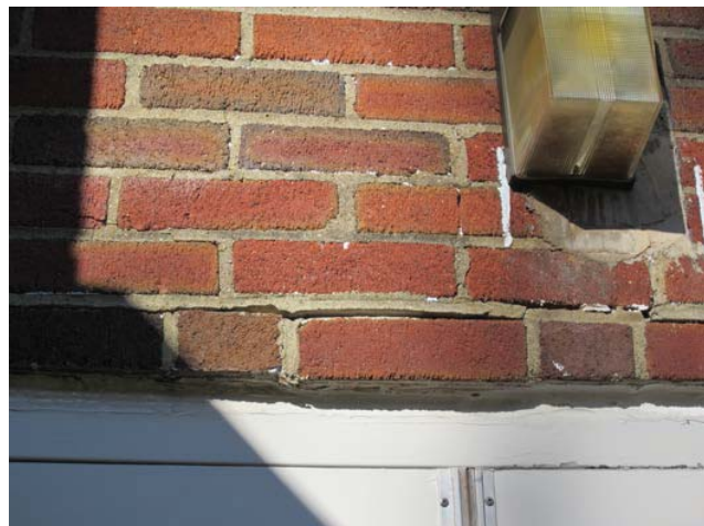
Figure 4: Cracks and open joints in mortar, masonry movement above doorway
