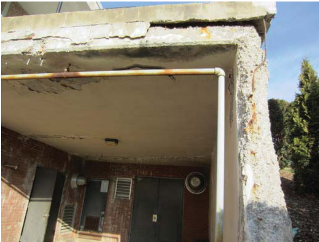
Figure 7: Concrete deterioration at service entrance
