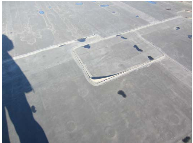
Figure 8: Seam separation between roof membrane materials (typical)
