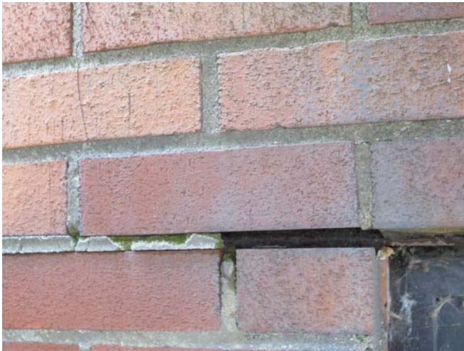
Figure 5: Window lintel corrosion cracking masonry and mortar joints
