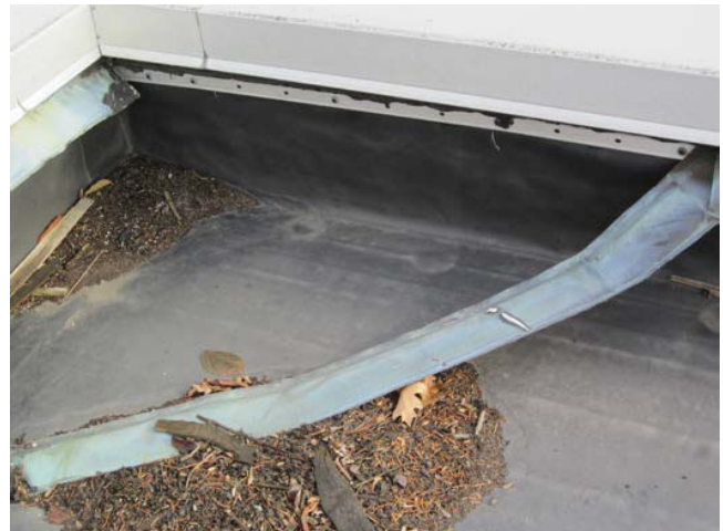
Figure 6: Loose copper flashing at roof
