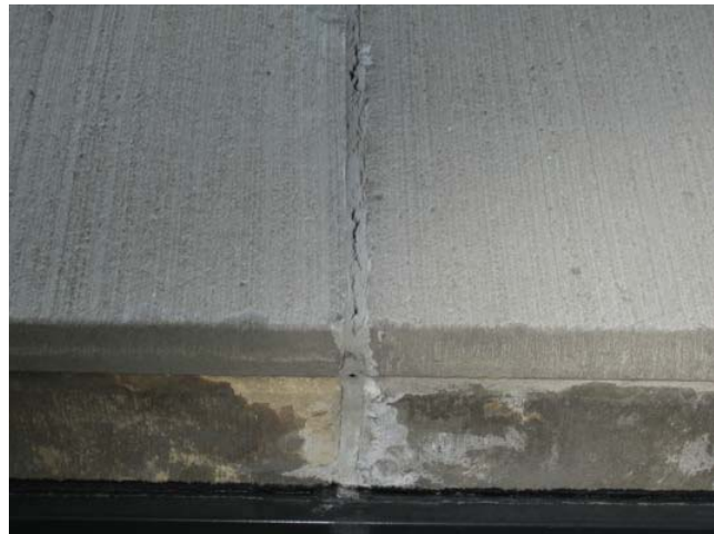
Figure 2: Sealant failure between precast panels
