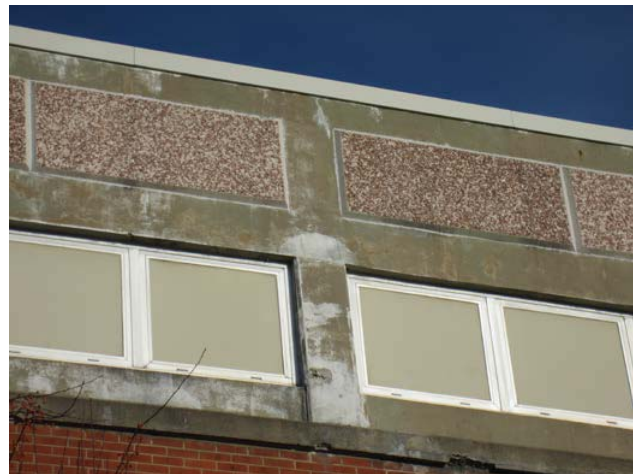
Figure 2: Concrete cracking and spalling
