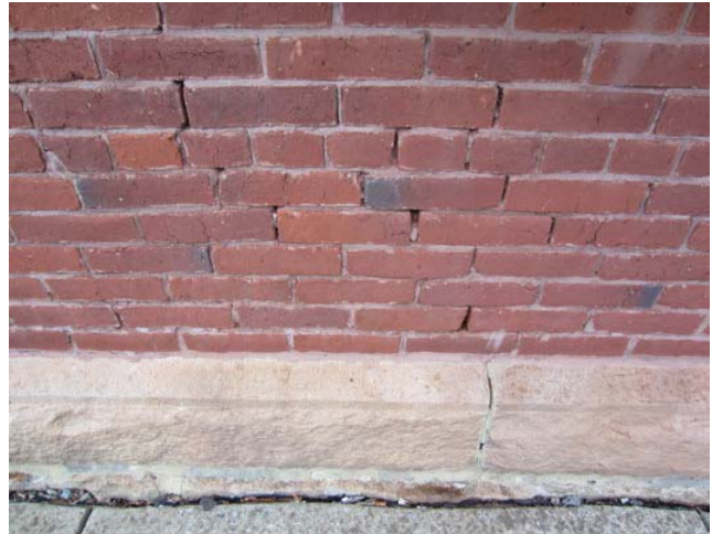
Figure 2: Cracks and open joints in exterior masonry
