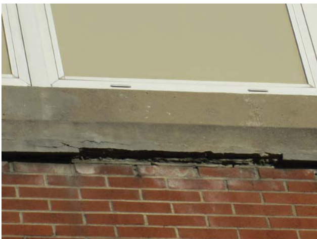
Figure 3: Concrete spalling and reinforcement corrosion
