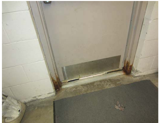
Figure 6: Hollow metal frame corrosion
