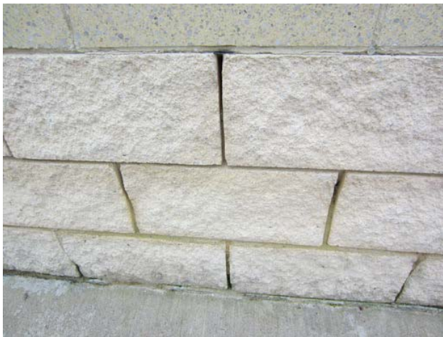
Figure 3: Mortar deterioration on north facade
