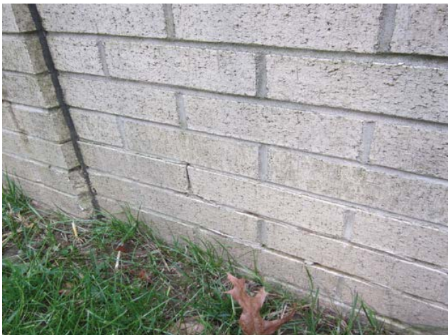
Figure 3: Cracked brick masonry
