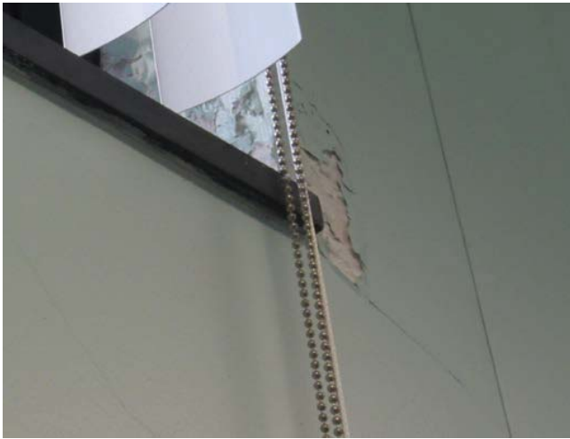
Figure 5: Water damage at window opening
