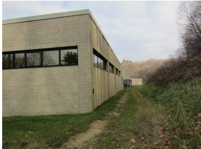
Figure 2: Southeast corner of building, site of past moisture infiltration into building.
