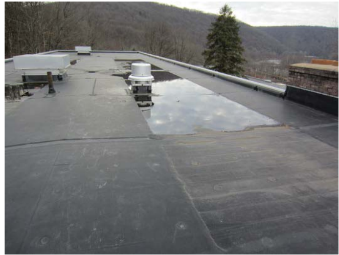
Figure 6: Water ponding on membrane roofing
