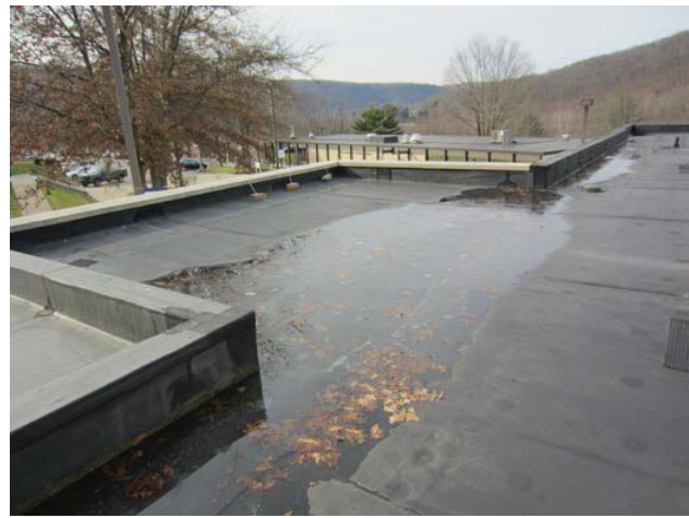
Figure 4: Rooftop water ponding
