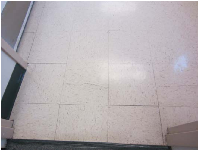
Figure 5: Cracks in vinyl composition floor tile
