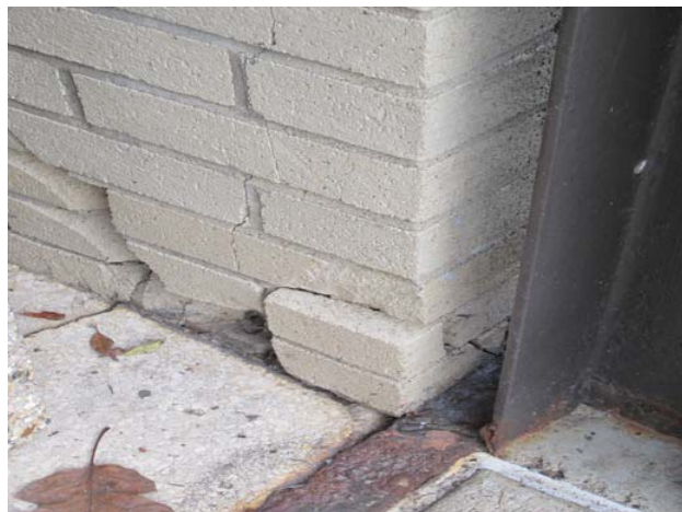
Figure 4: Cracked and broken brick masonry and steel corrosion
